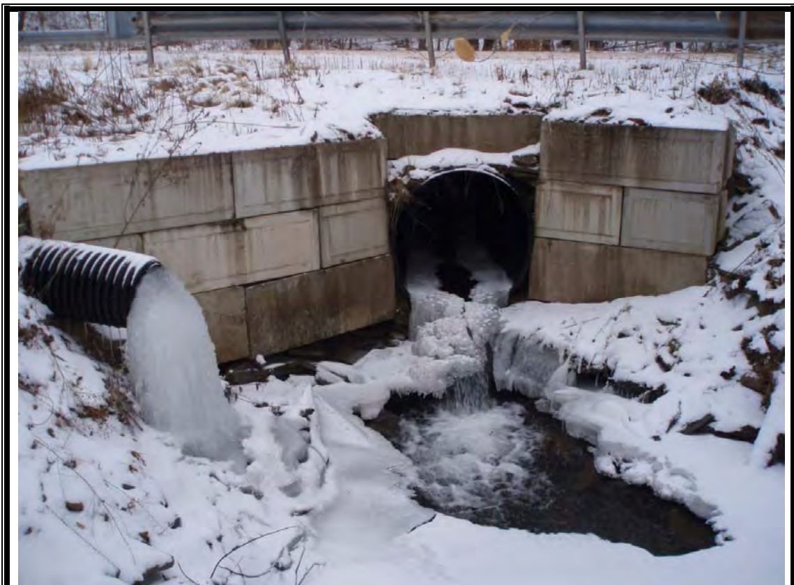
Photo 1: Looking upstream from right streambank at culvert outfall and failing head walls.
