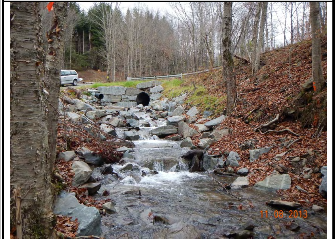
Photo 6: Looking upstream from bottom of project at step pools and culvert outlet protection.
