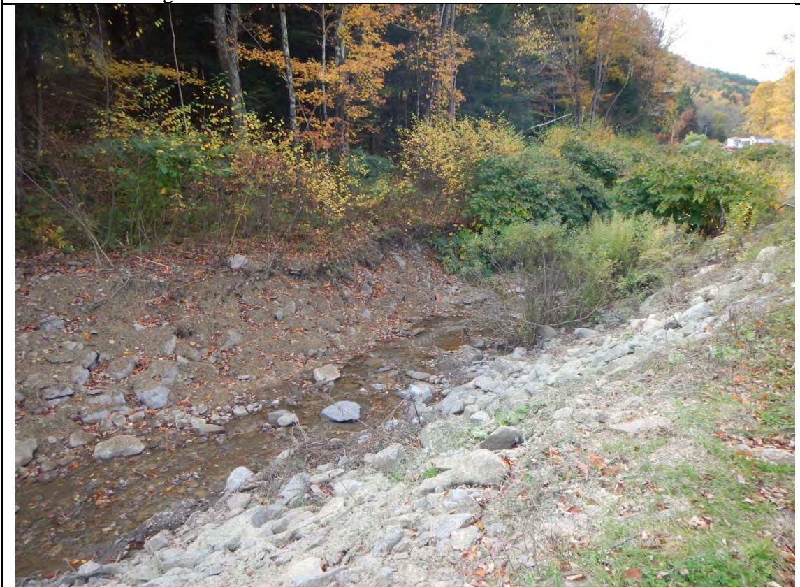
Photo 4: Looking downstream after construction at hardened riffle and rip rap along the toe of left streambank
