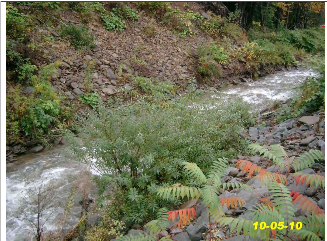
Photo 3: Looking downstream at left streambank erosion.
