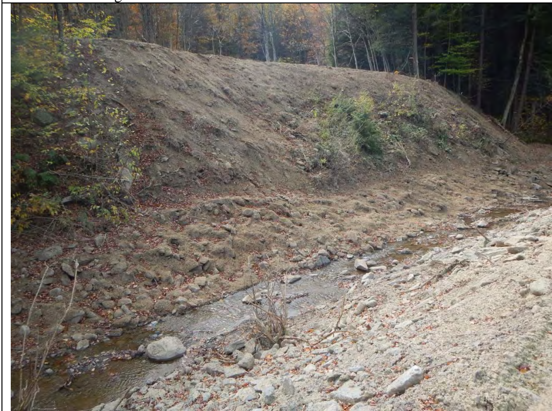
Photo 2: Looking downstream after construction at rock rip rap along the left toe of streambank.
